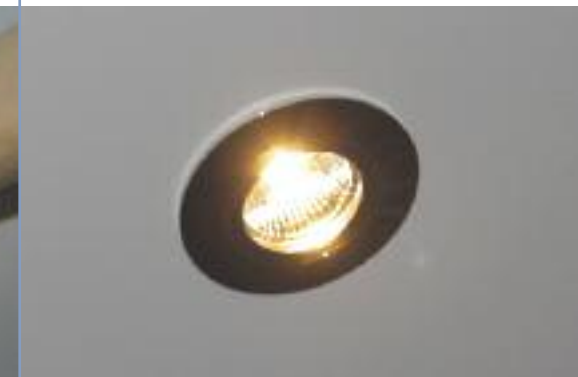
Fertig eingebautes Downlight Completed built-in spotlight
